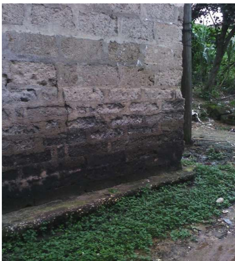
Figure 2: Building Foundation Exposed by Flood in Ayadehe Community Source: Field Research (2018)
