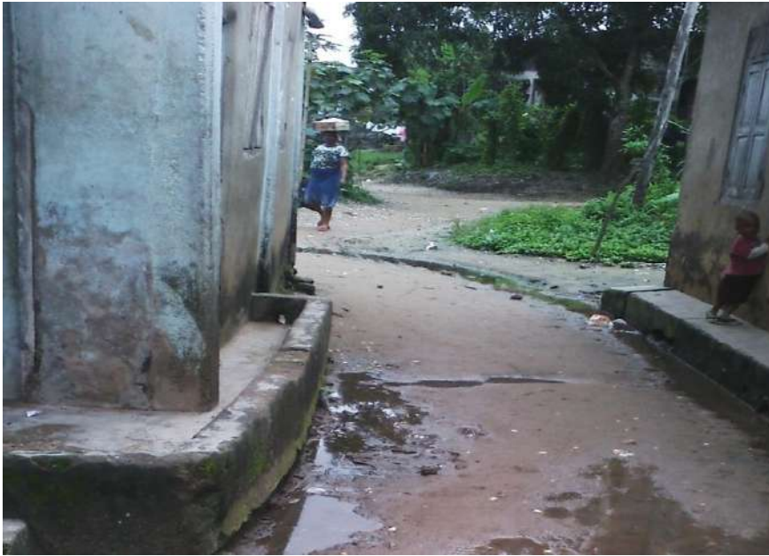
Figure 4: Raised slaps constructed round the buildings using a concrete mix of shells, gravels and cement to safeguard the foundation of a buildings in Akpaekpeneton Community. Source: Field Research (2018)
