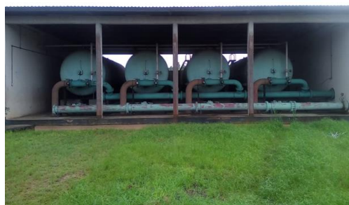
Plate III: Water Treatment Plant in Akwa Ibom State
