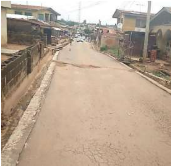
Plate 1: Deplorable road condition
